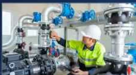
Pumps, Valves & Flow Control Systems
