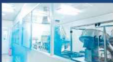
HVAC, Clean Room & Environmental Control Systems
